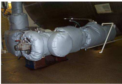
Figure 1 - Typical Inditherm Removable Jacket Heaters on a Pump
